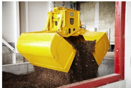
Plant-based fuel for the biomass boilers Tangiers plant
